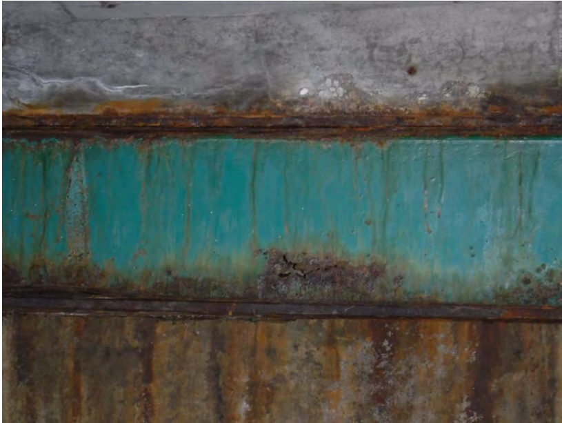
West Abutment, 2 nd Diaphragm from South Edge, Hole
