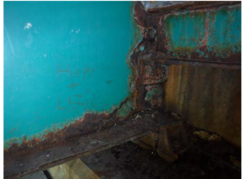
West Abutment, 2 nd Beam from North Edge, Typical Corrosion
