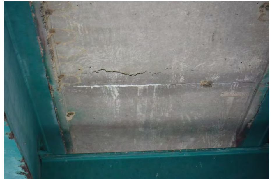
Superstructure, 1 st Bay from South Edge, Cracks
