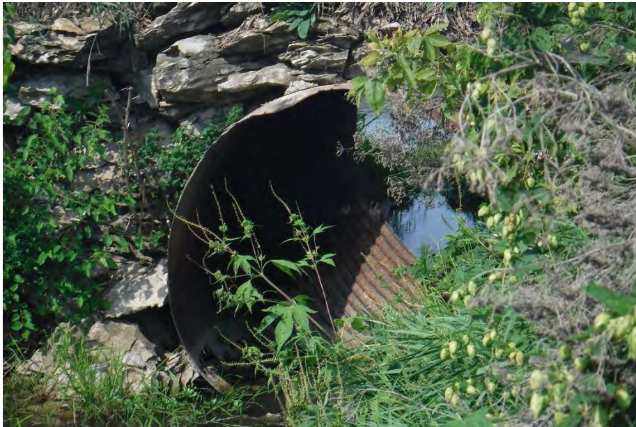
Failed North Barrel
