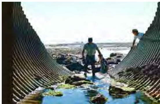
This aluminum structural plate pipe has handled tidal ocean waters under U.S. Highway 1 at the Bay of Fundy in Maine since 1966.
