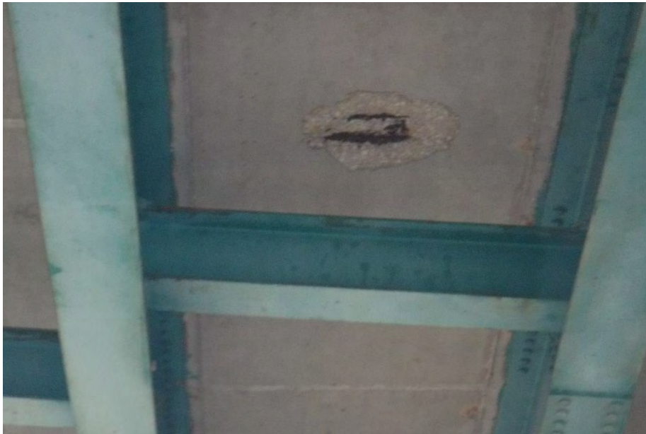
SPALL IN DECK CENTER SPAN
