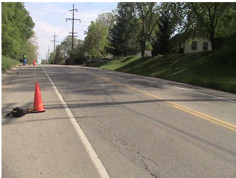
Figure 4. Sample Photograph of an Inspection Unit and Equipment Layout
