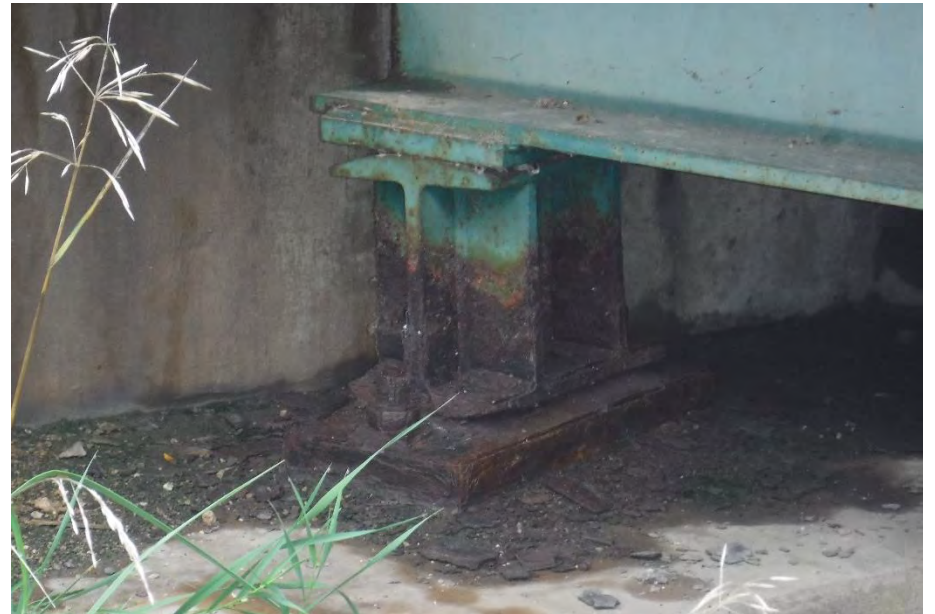
RUSTED BEARING NORTHWEST CORNER
