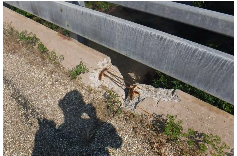
DAMAGED CURB OVER PIERS (TYPICAL)
