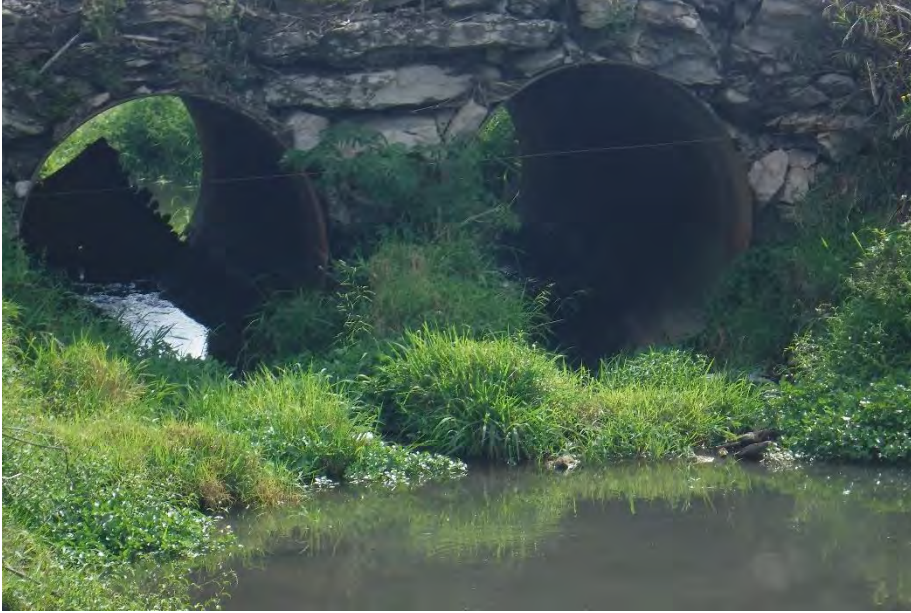
East End of Culverts – Note Failed North Barrel
