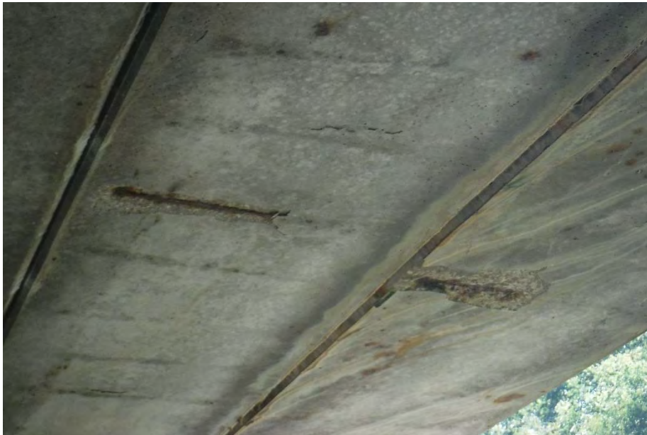
SOUTH SPAN SPALLING
