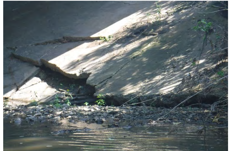
SOUTH SLOPE WALL CRACK
