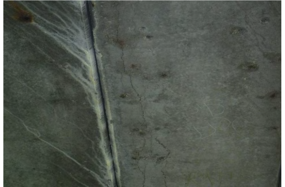
SOUTH SPAN BEAM CRACKING
